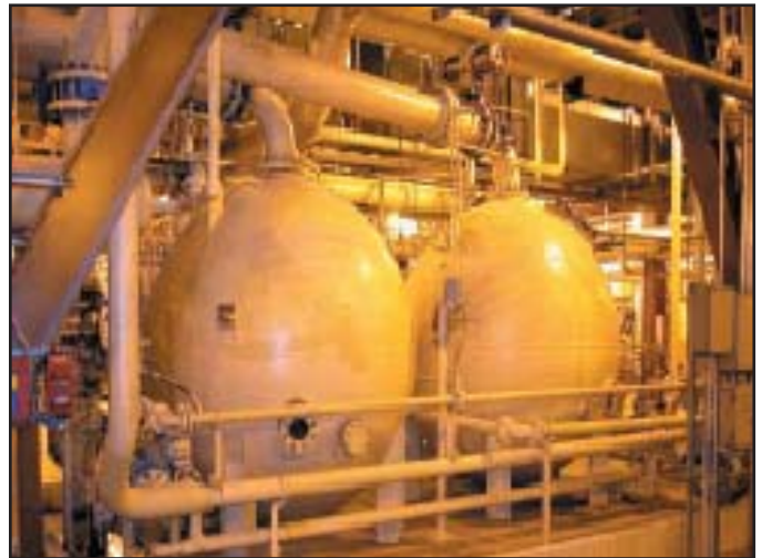
These condensate polishers purify water so well that it won't even conduct electricity. High purity is required to minimize corrosion in the closed-loop steam generation/condensation system.
