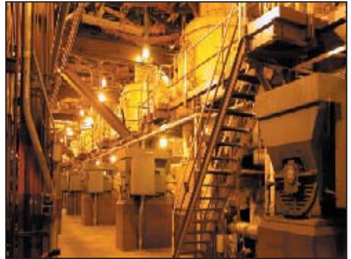
Massive pulverizers crush the incoming coal to a fine powder, the consistency of talcum, so it can be air-conveyed into the boiler furnace.
